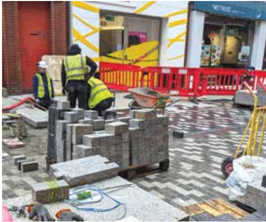
Workers paving a newly pedestrianized street in Dublin. Photo credit: Judy Minot
